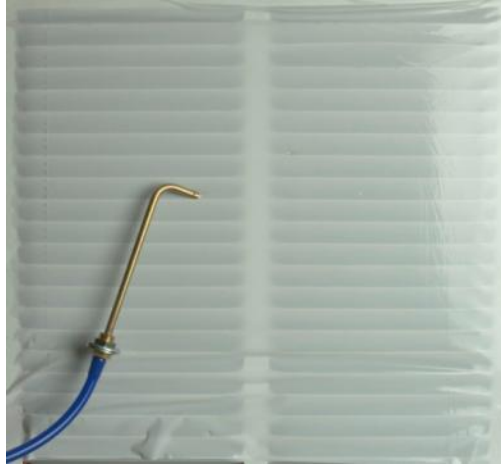
Figure 16: Insert the blue tube into a supply register closest to the air handler
