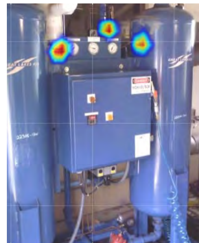
Figure 1. With portable acoustic imagers, technicians can quickly locate compressed air leaks simply by pointing the device at an asset or system or scanning a large area – from a safe distance, with the line still running, and no matter how noisy the plant.
