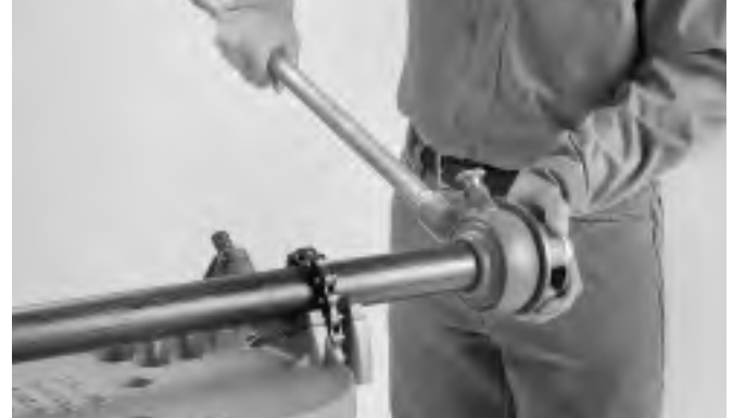
Figure 3 – Sliding Threader On Pipe
