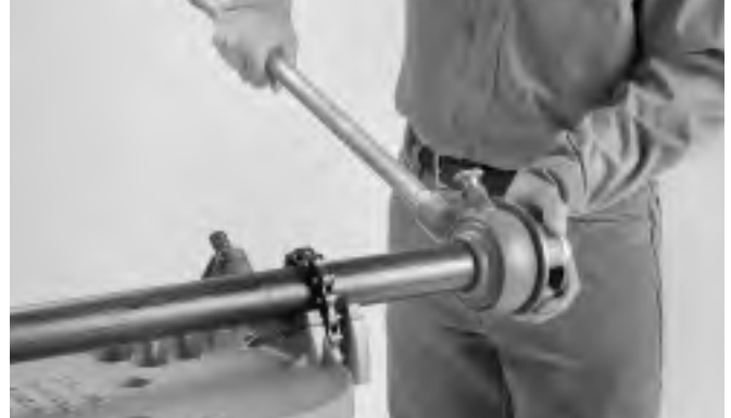
Figure 3 – Sliding Threader On Pipe
